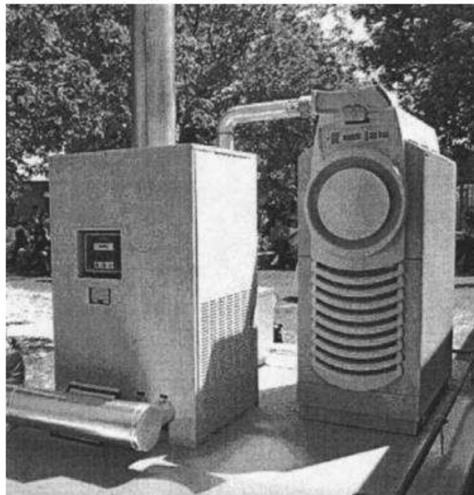
Figure 41. Microturbine in a combined heat and power installation.
